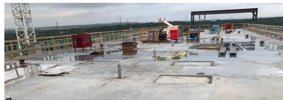
Photo 2: This is a before picture of what Westover Hills Baptist Hospital looked like at the beginning of the construction process.
