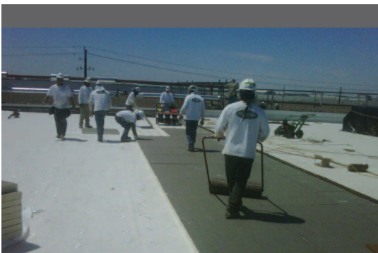
Chamberlin installed 10 inches of insulation atop Houston Food Bank's freezer and cooler.
