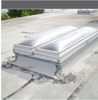
The existing skylights were in need of replacement.
