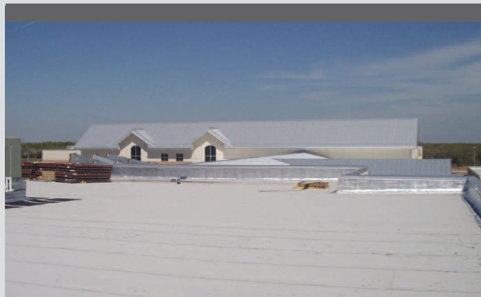
Following the "keep it off the roof" concept, this modified bitumen roof system has provided good service since 2003.
