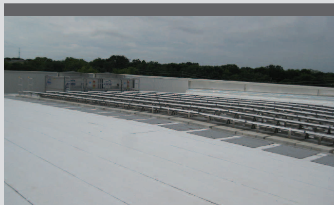
This roof supports a ballasted tray system for a solar array. The roof was replaced prior to installation of the solar system.
