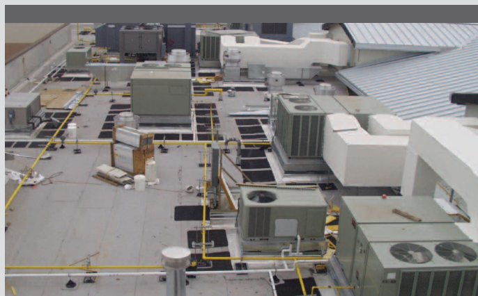
This roof is the platform for mechanical equipment, ducts, piping, vents, etc., all of which need to be considered during design.
