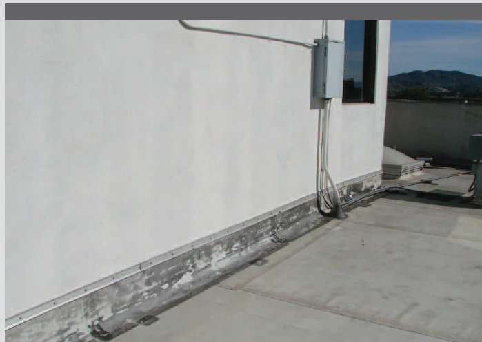
The roof membrane terminates to the face of the cement plaster without a weep screed at the plaster base. As installed, the plaster system will drain out underneath the roof system.
