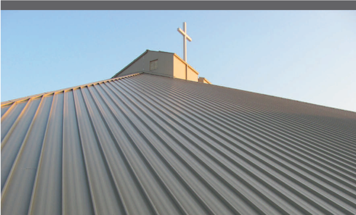
The new metal standing seam roof of Great Hills Baptist Church in Austin, Texas.
