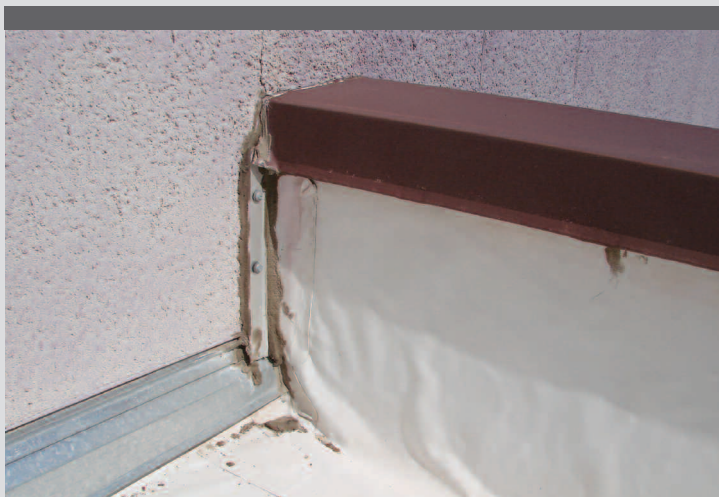
This photo shows no continuity between EIFS, roofing, flashing, and coping. EIFS should be flashed around parapet with an added weather seal and weep system.
