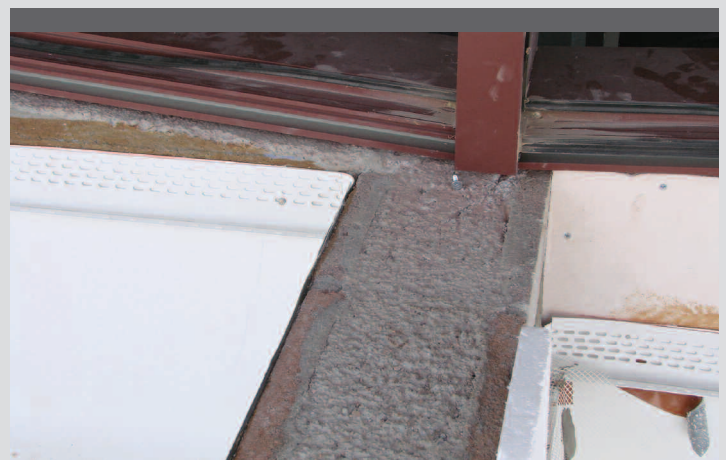
This lack of continuity between the sill of glazing, EIFS and roofing at parapet walls creates potential points of water infiltration.
