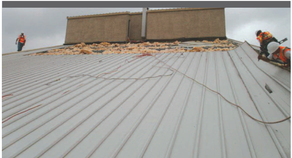
Chamberlin workers remove the old roof of the sanctuary in preparation for the new metal roof system.
