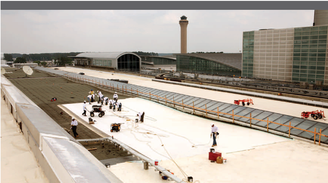
An expansive look at the 220,000 sq. ft. Terminal D re-roofing project in progress.
