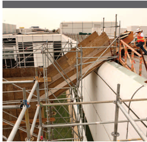
A 60 ft. tall, free standing garbage chute was engineered to handle 220,000 sq. ft. of demolished roofing material.
