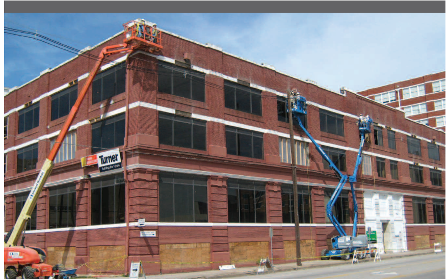
Chamberlin's scope of work on the Dallas County Community College District's office involved the complete restoration of the building's exterior, interior and roof.
