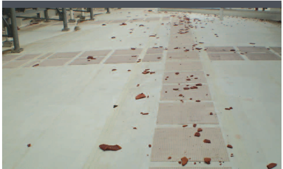
Debris scattered across roof at the Memorial Hermann Hospital Campus as a result of heavy winds from Ike.
