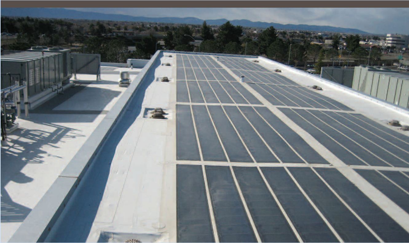
Building Integrated Photovoltaic System (BIPV).
